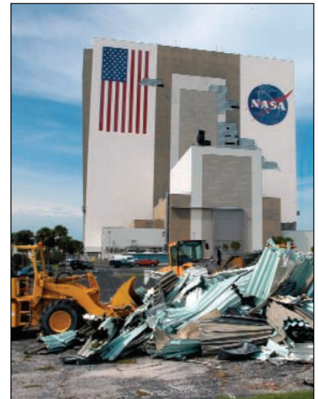
Space scuttle. Hurricane Frances shredded the walls of a Kennedy Space Center building used to assemble shuttle parts.
